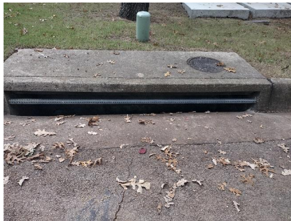
Safety cross bars in drainage inlets
