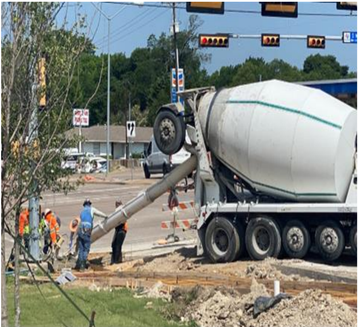
Concrete Placement for Curb Ramp at S. Main St. and E. Danieldale Rd.
