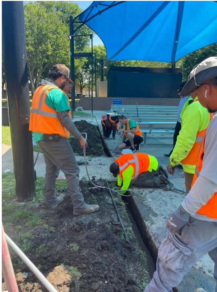
Amphitheater Lighting Project
